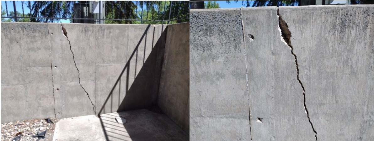
Department retaining wall on North side of the building before repair, June 23, 2022
