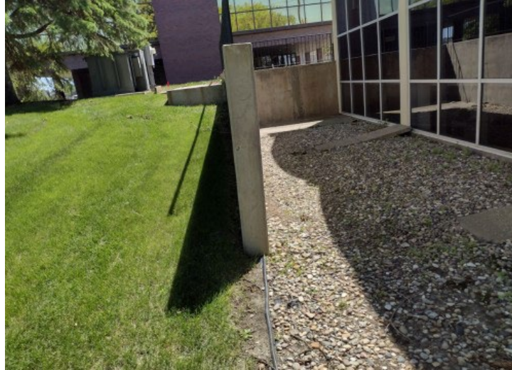
Department retaining wall North side of the building before repair, June 23, 2022
