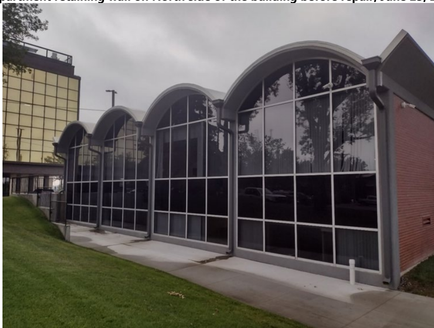
Department retaining wall North side of the building after wall repair, July 23, 2024
