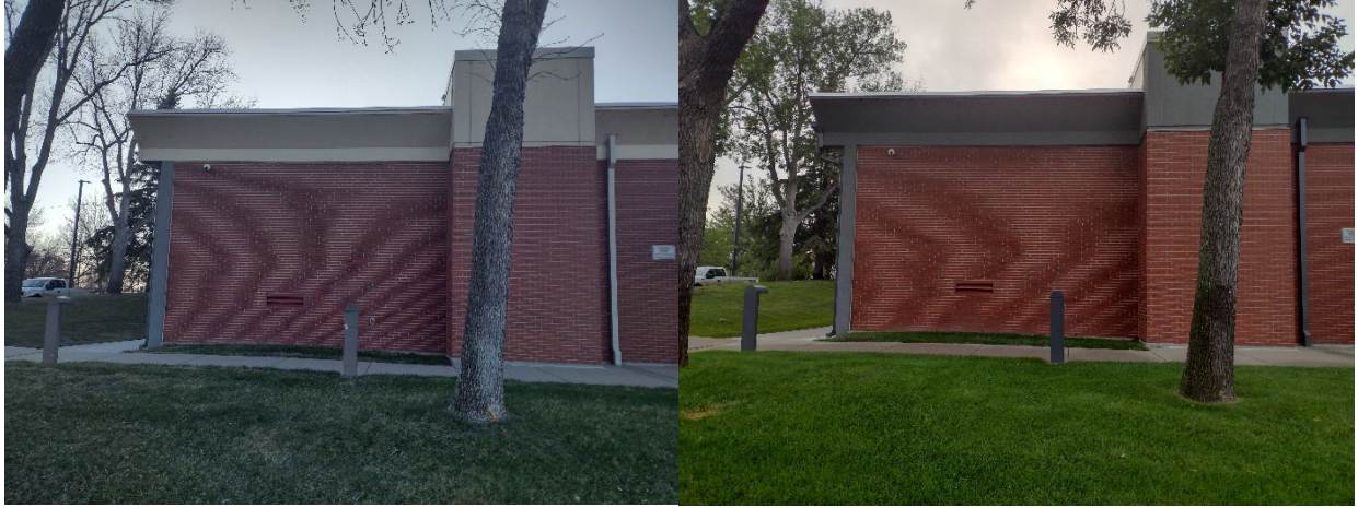
West Side of the building before painting, April 23, 2024 and after painting, July 25, 2024
