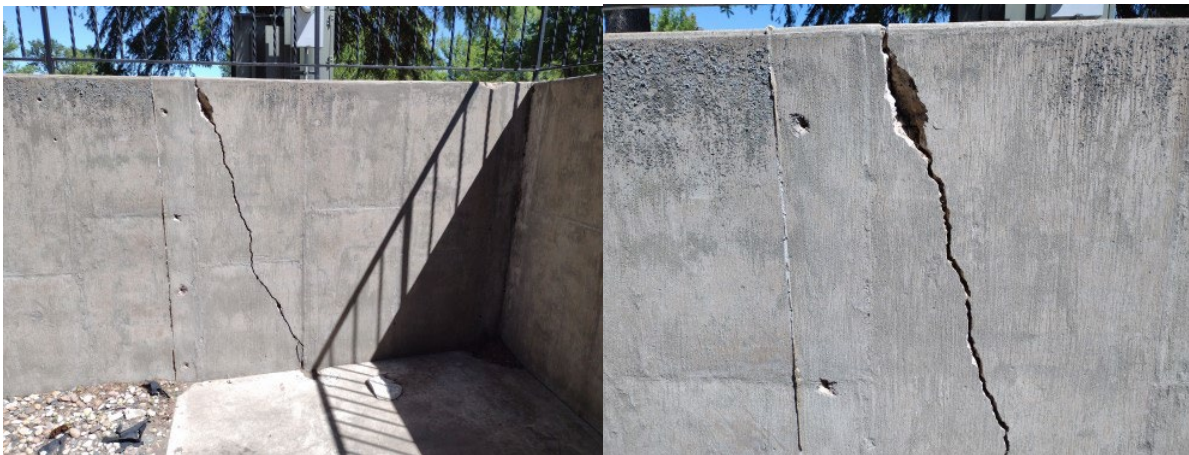
Department retaining wall on June 23, 2022. North Side of the Building Photo credit: Rick Owings
